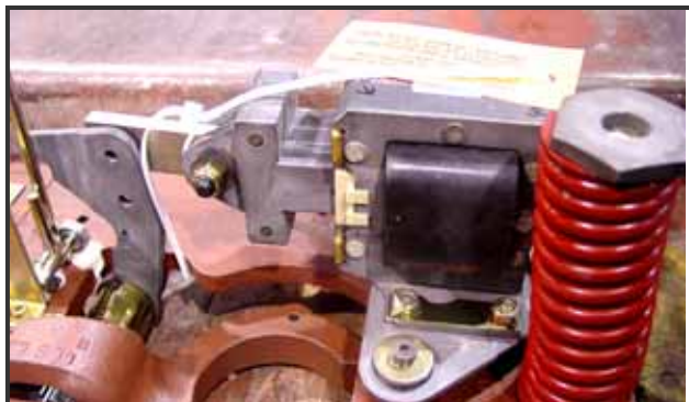
Picture A: Cable strap holds the plunger into the solenoid frame of a new brake.
